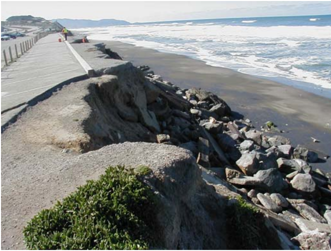
South Parking Lot Erosion, 2000
