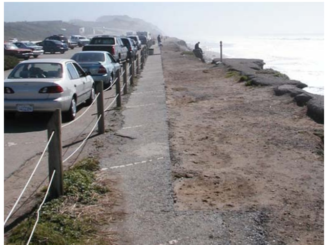
South Parking Lot Erosion, 2005
