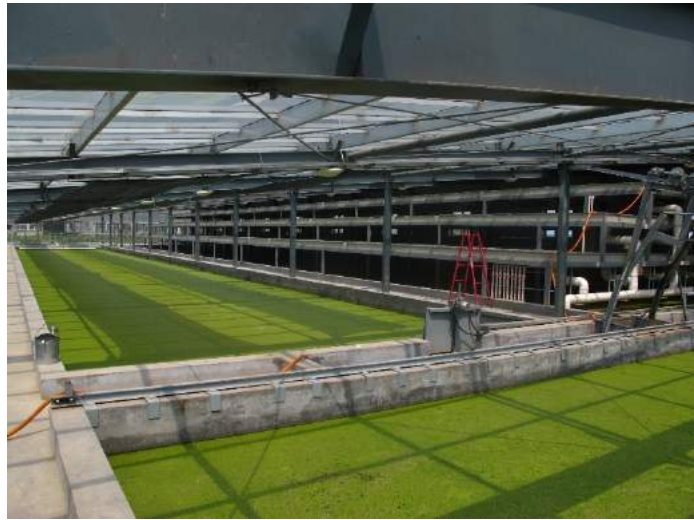
Duckweed-based wastewater system at Qingdao Institute of Bioenergy and Bioprocess Technology, Chinese Academy of Sciences, China
