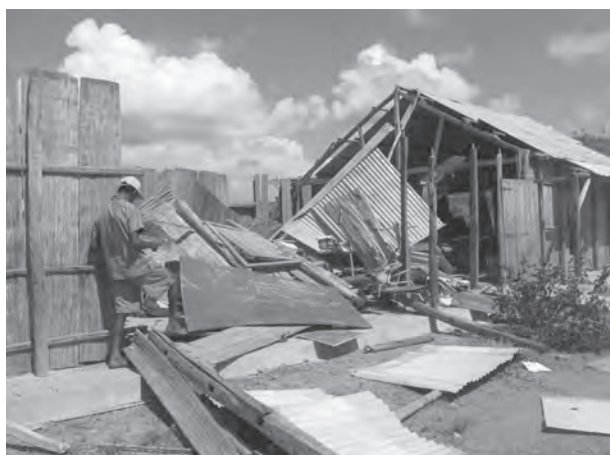
Fig. 4: The public primary school in the Lanonana village, near Andriantantely forest, Brickaville District, damaged by Cyclone Giovanna in February 2012. (Photo: Hery Randriahaingo)
