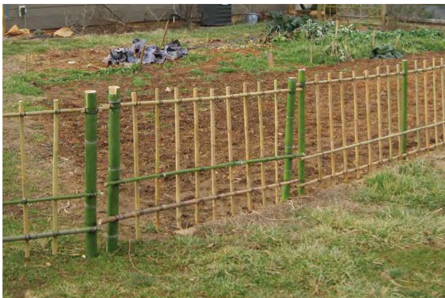
Finished sections are set in a row by slipping the larger outer poles over rebar sunk in the ground.
