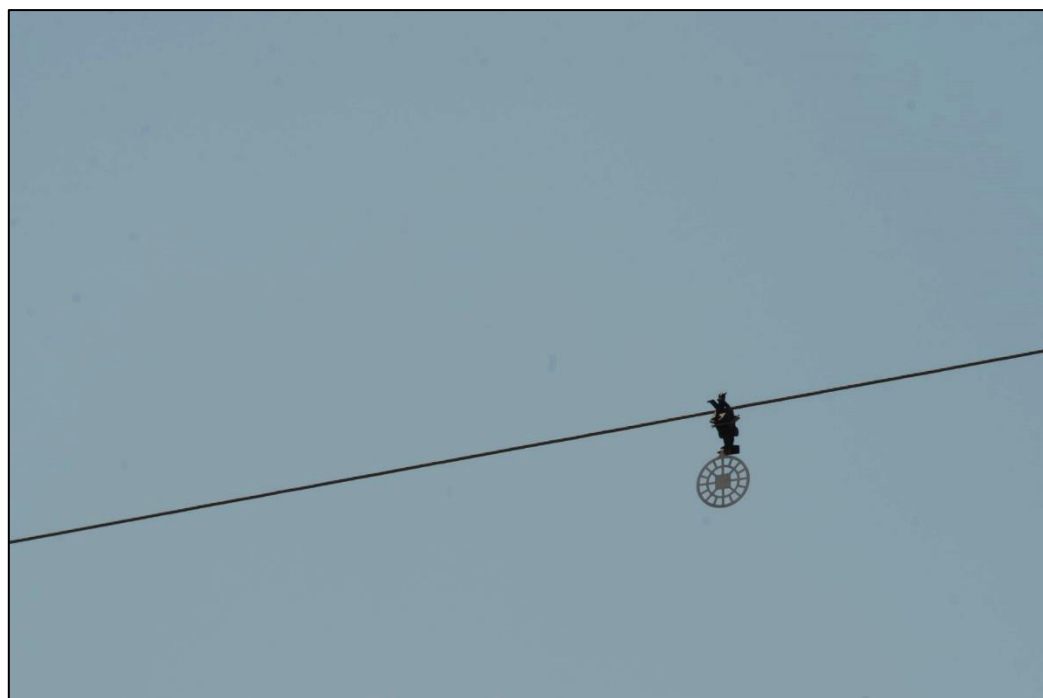
Figure 11: Bird flapper observed on the electrical wires in the project area
