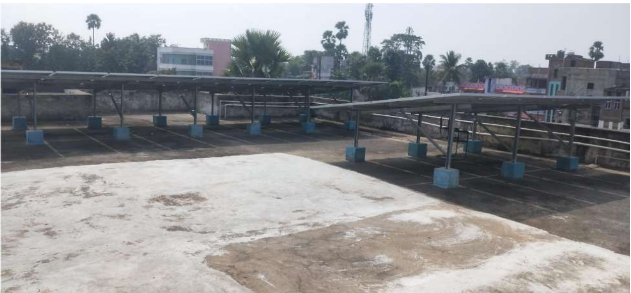
Fig- Solar PV panel system present on the roof of Arts block
