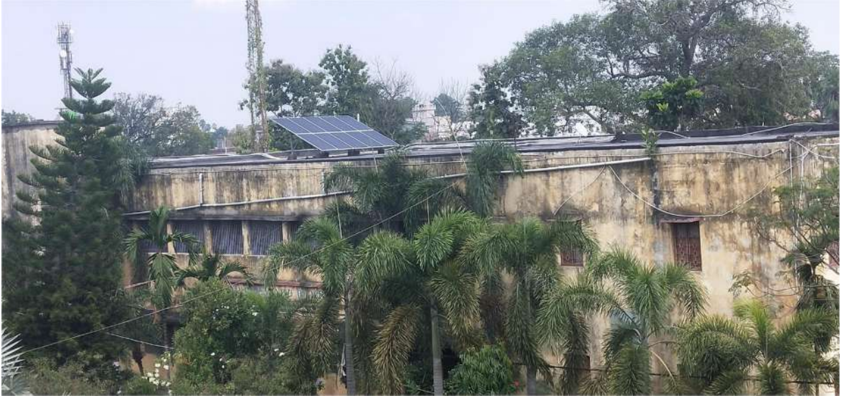
Fig- Solar PV panel system present on the roof of Administrative Block
