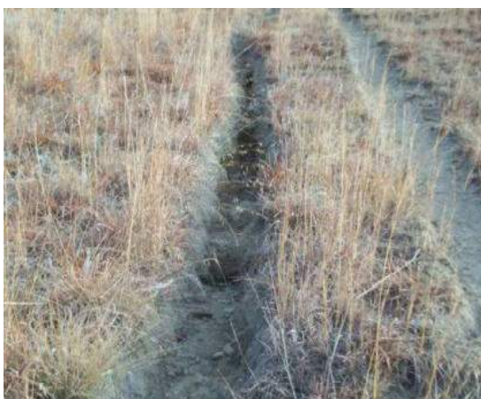
Erosion channels starting to form along existing cattle tracks
