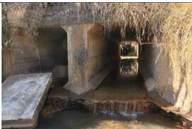
Photo 12: The culvert system of Pierre Road has been placed above the natural channel morphology of the watercourse resulting in water damming up before the culvert.
