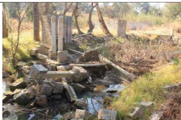
Photo 15: Building rubble used as a dissipator below the head cut created by the culverts of the bridge.
