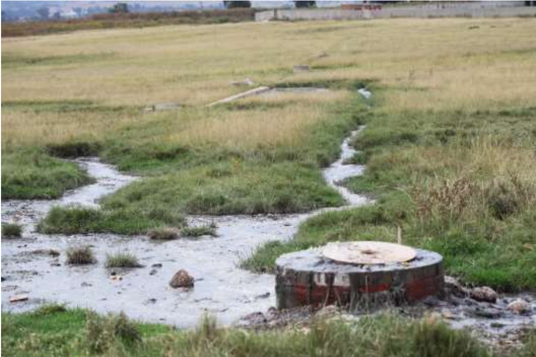
Photo 11 Sewage leak at the tributary at the southern part of the site. Photo: R.F. Terblanche.
