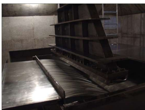
FIG. 3. Under beam wastewater reactor.
