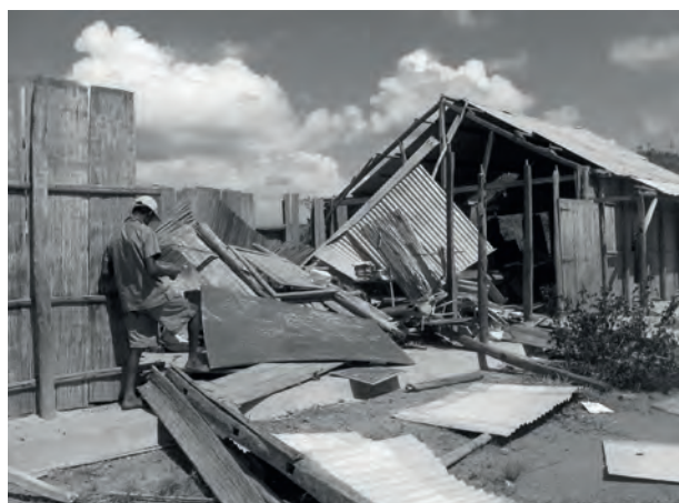
Fig. 4: The public primary school in the Lanonana village, near Andriantantely forest, Brickaville District, damaged by Cyclone Giovanna in February 2012. (Photo: Hery Randriahaingo)
