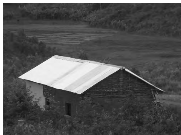
Fig. 6: The primary school in the village of Ranomainty, Didy Commune, in Nov 2012, repaired following damage by Cyclone Giovanna. (Photo: Lucien Randrianarimanana)
