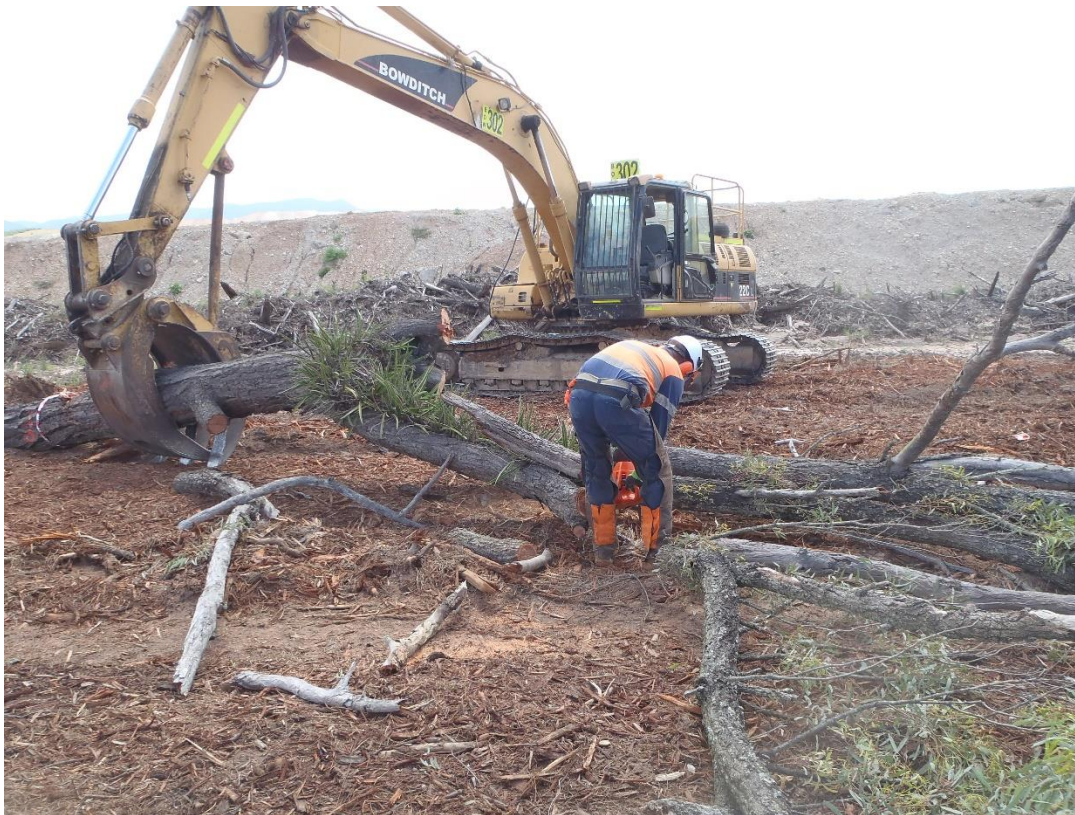
Figure 3.1 – salvage of tiger orchid ensuring maximum amount of original host tree maintained
