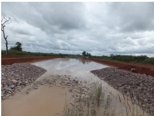
Figure 72: Example of Sediment Ponds
