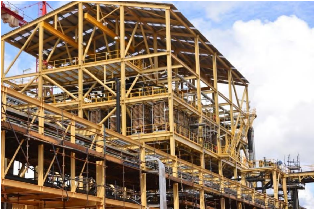
Figure 2.7: The Kwale Mine's Wet Concentrator Plant (WCP)
