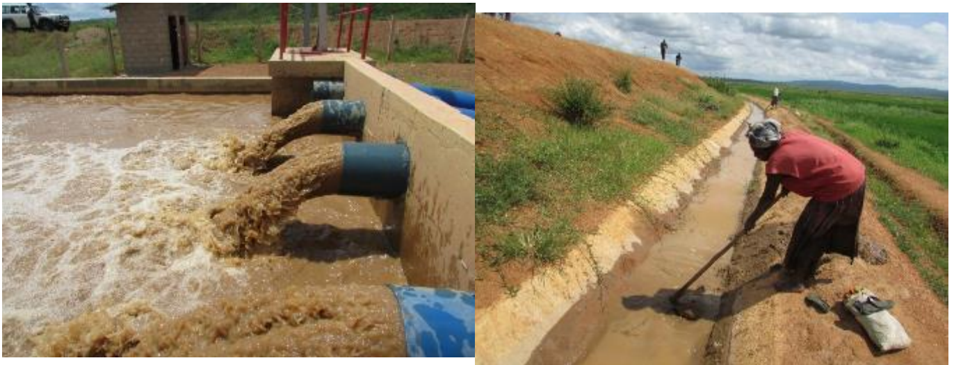
FIGURE 2- 55 PUMPING STATION AND SILTED CANALS IN THE BUGESERA AGRICULTURAL DEVELOPMENT SUPPORT PROJECT (PICTURES: APRIL 2017)
